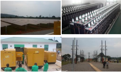
A 600kW PV & 1MW diesel hybrid mini-grid set-up on Bugala Island by Kalangala Infrastructure services commissioned in Jan 2015
