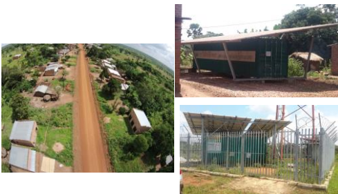
22.5kW PV System Installed by Kricher Solar in Uganda to supply the village and a telecom tower
